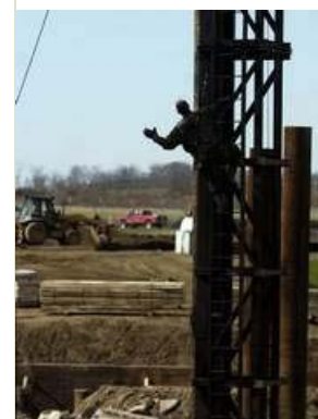
A construction worker signals his coworkers as he climbs a pile driver while a crew sets a pile into the device Thursday afternoon off Irving Wick Drive in Heath. The piles are for a bridge that is part of the James Parkway extension. (Matthew Berry, The Advocate)
